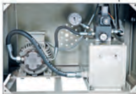
Hydraulic power pack inside
